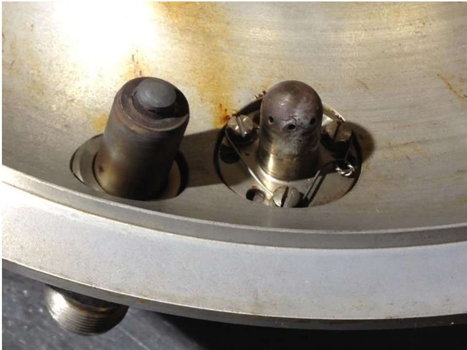
Burner head and igniter plug
